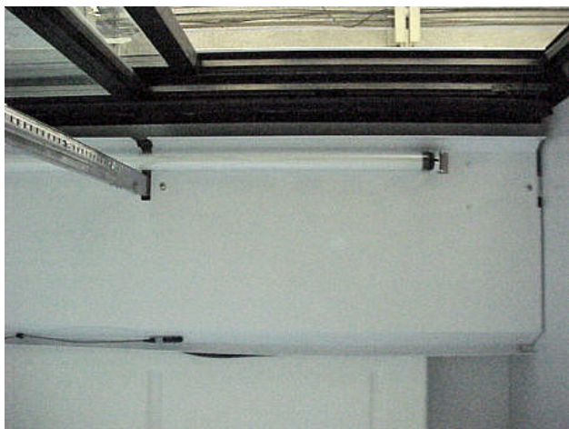
Chamber ceiling with lighting fixture -This must be removed to gain access to the evaporator coils.
