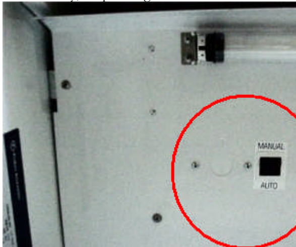
Figure 10. condenser fan switch (located on chamber ceiling)
